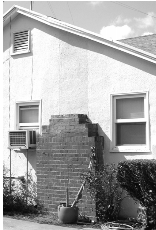
Figure 35 - Photo showing damaged chimney removed. Note that the fireplace is now not functional.
